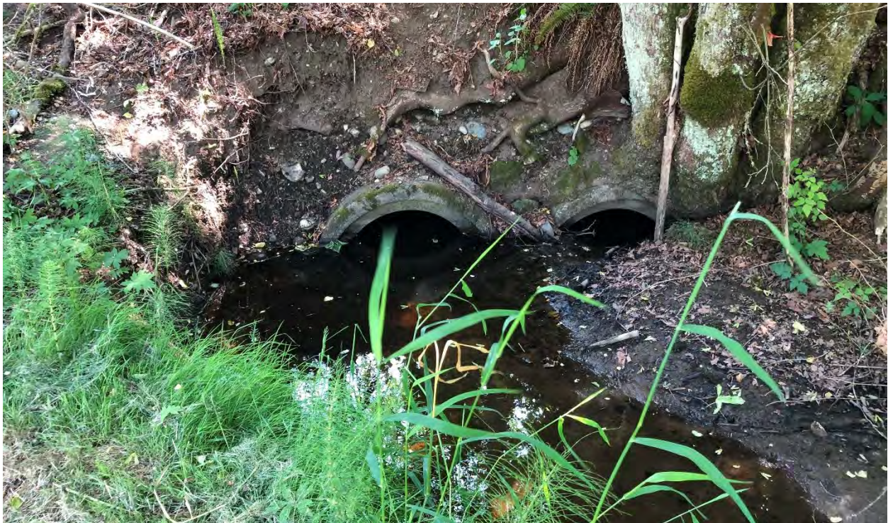
Photo 5. Viewing downstream (east) to the inlets of the culverts under the abandoned railroad berm. The culverts are partially plugged with sediment (May 30, 2019).
