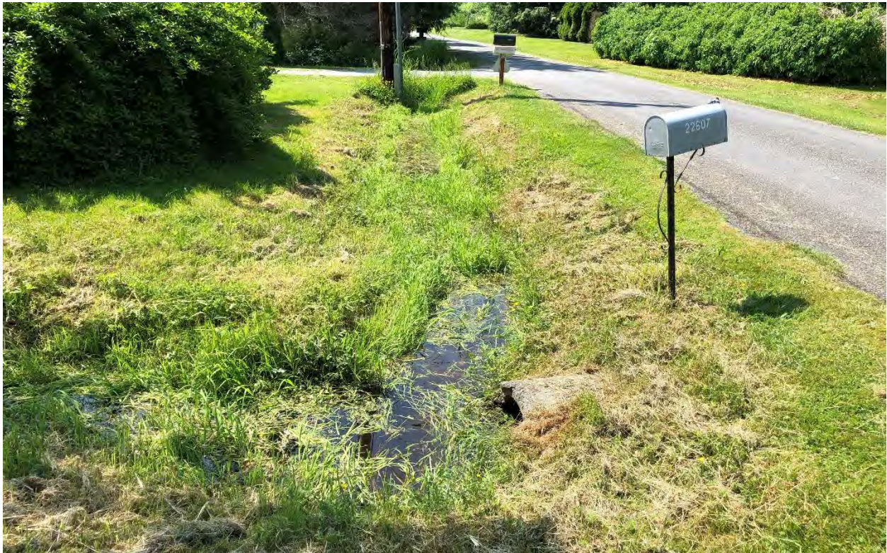
Photo 6. Viewing upstream (south) along the Hull Road ditch. The culvert near the mail box is the culvert that carries the stream under Hull Road. The stream exits the left side of the photo (May 30, 2019).
